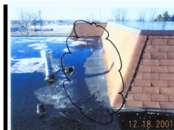
Note EPDM membrane shrinkage pulling flashing membrane away from shingle roof. Bottom course of shingles are almost horizontal.
